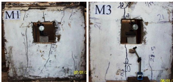
Figure 2 Crack Pattern of M1 Figure 3 Crack Pattern of M3
