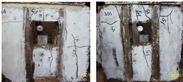
Figure 4 Crack Pattern of M4 with longitudinal GFRP Laminates Figure 5 Crack Pattern of M6 with longitudinal GFRP Laminates
