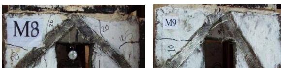
Figure 6 Crack Pattern of M8 with Diagonal GFRP Laminates Figure 7 Crack Pattern of M9 with Diagonal GFRP Laminates
