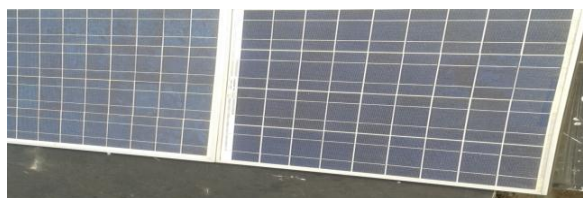
Fig.2 PV modules of Jain Irrigation in outdoor exposure
