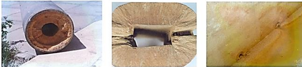
Fig.1 Deposit and scaling
