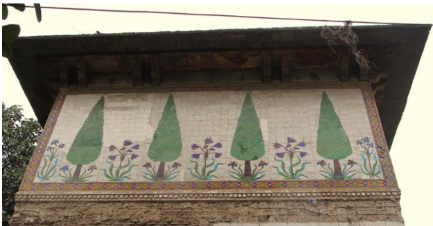
Plate.5 Partial damages on the Exterior of the Cypress tomb which is adorned with Cypress motifs in glazed tiles. Source: Photography by the author.
