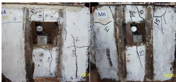
Figure 4 Crack Pattern of M4 with longitudinal GFRP Laminates Figure 5 Crack Pattern of M6 with longitudinal GFRP Laminates
