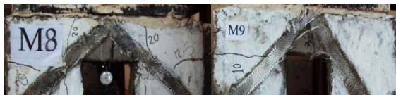
Figure 6 Crack Pattern of M8 with Diagonal GFRP Laminates Figure 7 Crack Pattern of M9 with Diagonal GFRP Laminates
